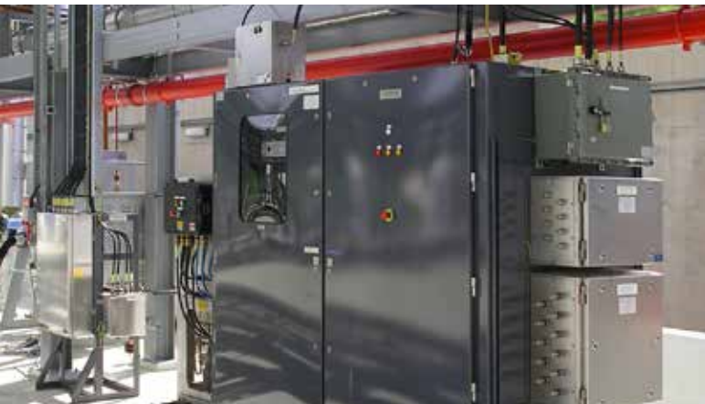
Exp Electrical Panel at BAE
